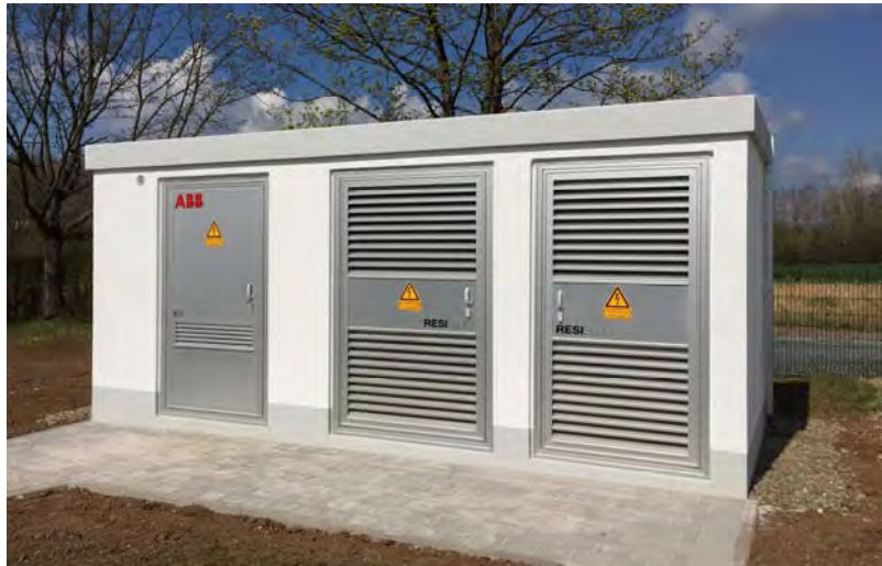
HITACHI ABB POWER GRIDS © Hitachi ABB Power Grids 2020. All rights reserved
