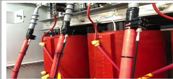
Figure 8: PD monitoring at a dry transformer using UHF PD sensors
